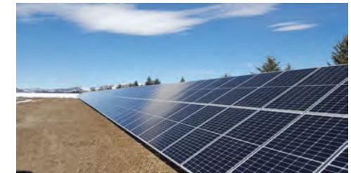
Hillside Ranch Irrigation - 99.74kW Bellvue, ID 2020
