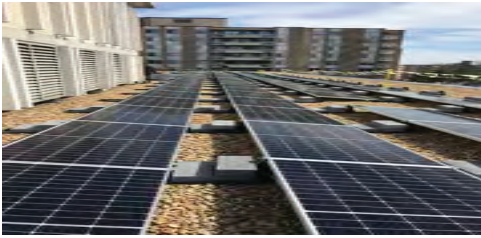
Van Ness Center Associates, LLC - 200.265 kW Washington, D.C. 2020
