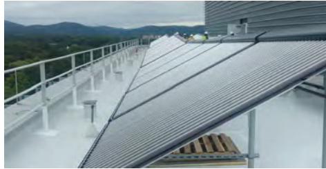
UVA Hospital - Thermal System Charlottesville, VA 2020
